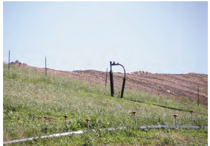
Gas to energy - Denton Landfill
