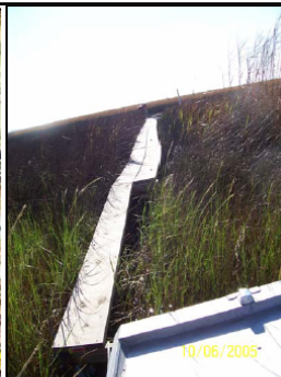
Figure 2: CRMS0434 boardwalk with missing board and warning sign post.
