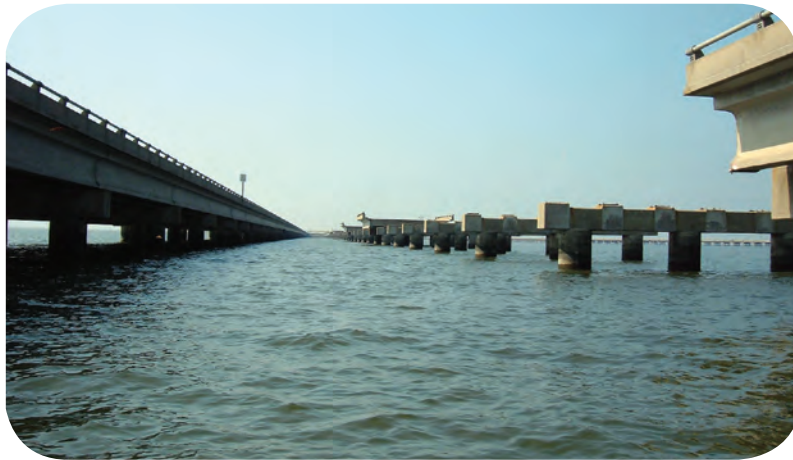
Figure 6. Sections of the Interstate 10 Twin Span Bridge, La., displaced by Hurricane Katrina's storm surge.
