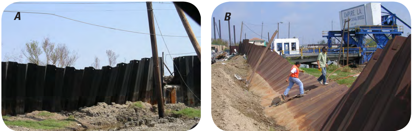
Figure 6. Rotational failure of the piling with possible toe movement (A), and total collapse of piling at Empire, La. (B), as a result of Hurricane Katrina in 2005.
