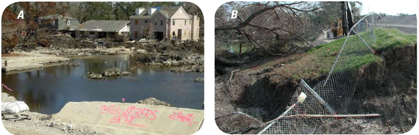
Figure 11. Failed concrete wall at the Metairie Outfall Canal (popularly known as the 17th Street Canal) breach (A), and horizontal translation of fence that used to be only 10 ft (3 m) from wall is now about 50 ft (15 m) away (B) resulting from the effects of Hurricane Katrina in 2005. Note the dark soft soil which formed a weak foundation for these structures.
