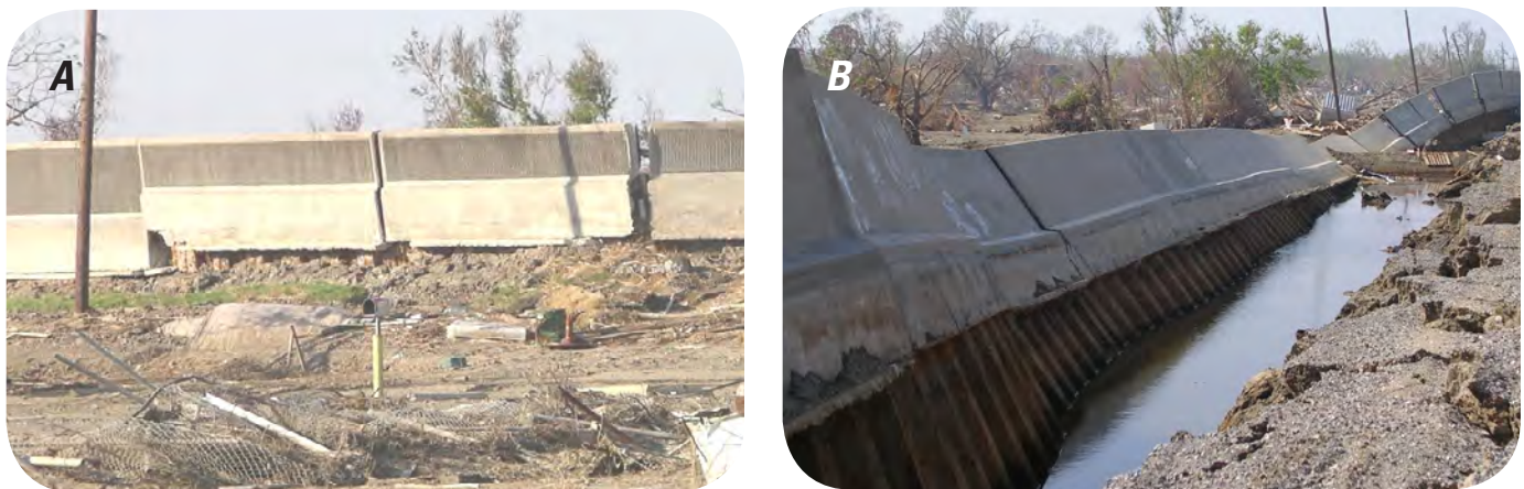
Figure 7. Failure of a concrete overwall; note that the underlying piling keeps the wall segments in place. Landward (protected) side (A), and water side (B).
