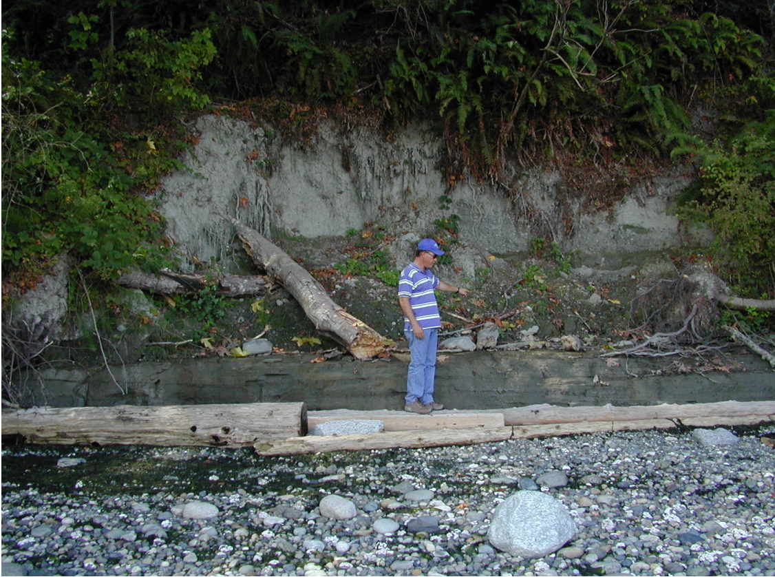
Figure 12. Small, unmapped landslide along the beach on the east side of the Colvos Passage. Note the color difference in the geologic units visible. Lower unit is a dense, layered silt/sand. Upper unit is less dense than the lower unit and is coarser sand with no visible layering (photograph: Jeffrey A. Coe, 2003).
