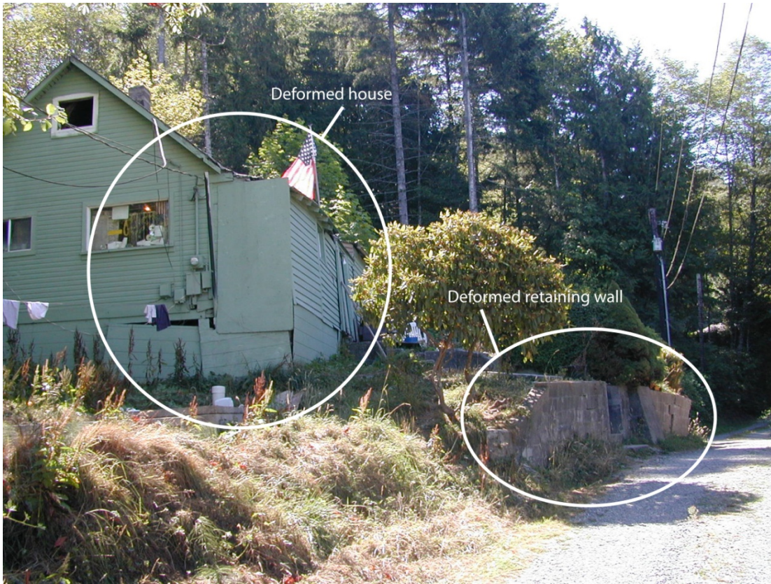
Figure 9. House and retaining wall on landslide 159 (see map) on the south side of Sinclair Inlet (photograph: Jeffrey A. Coe, 2003).
