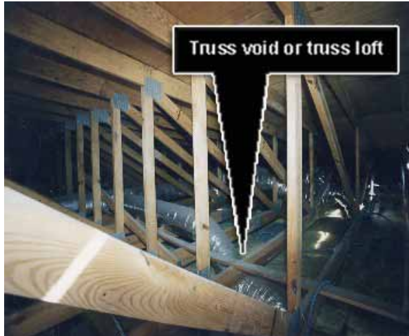
Figure 2. Truss loft with space for ventilation ductwork, wiring, etc. (Photo courtesy of National Fire Protection Association.)
