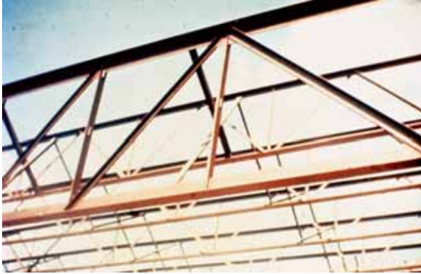
Figure C-4. Lightweight steel trusses. (Photo courtesy of Francis Brannigan.)
