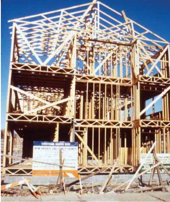
Figure 1. Typical lightweight truss construction. (Photo courtesy of Vincent Dunn.)
