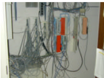
Unsecured and exposed communications wiring
