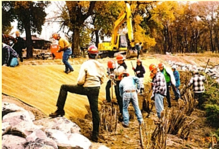
Coconut Fabric (Coir) Erosion Control Placement, with willow root ball planting and seeding, Carson River, 1998
