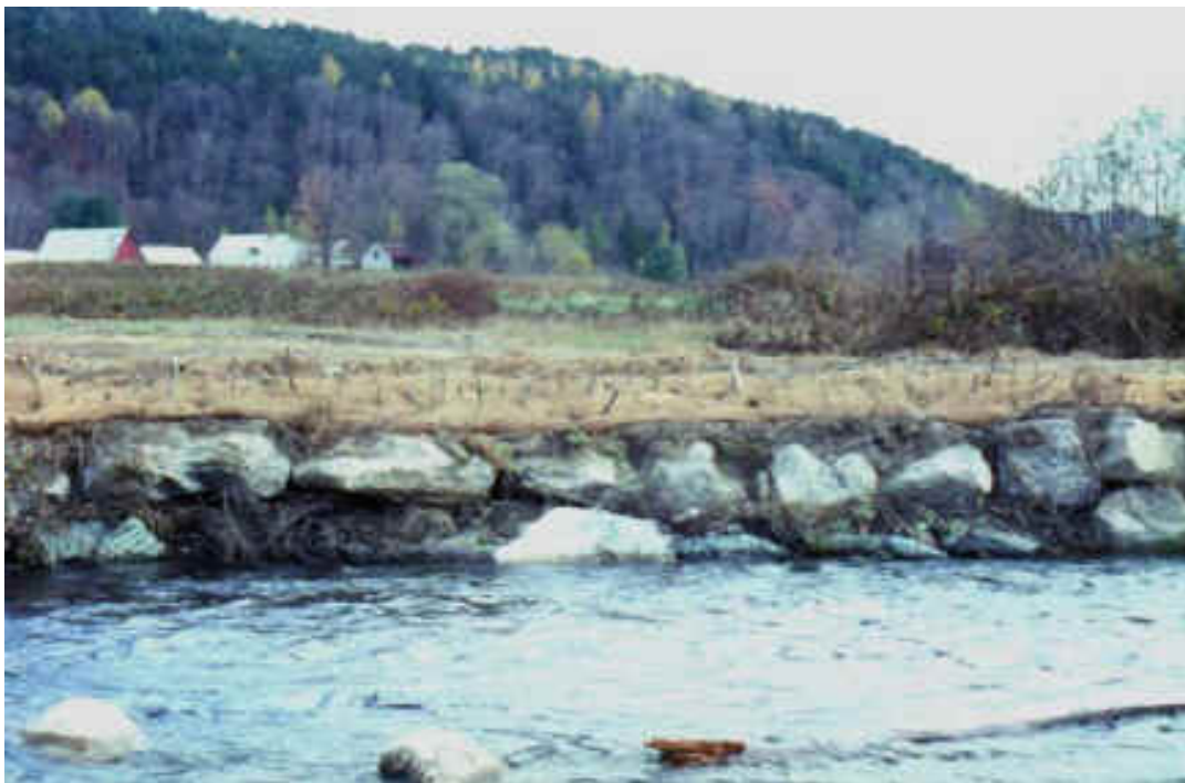
Rock revetment with brush layers, coir fabric and live stakes immediately after installation
