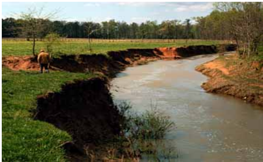
Before restoration – close up view of eroding streambank (1998).
