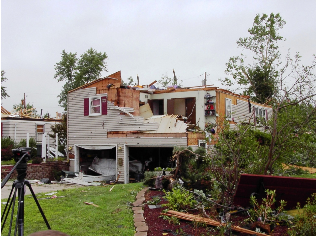
Tornado damage in Griffith, IN. Photo by Tim Halbach
