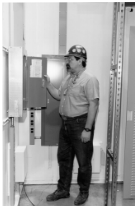
Larry Schultz of West Elsdon Electric checks an electrical box that has the proper work space allowance in front of it.
