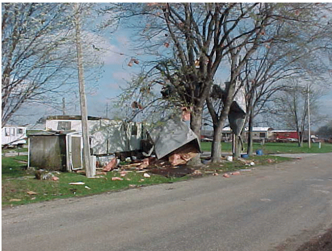
Roof of mobile home was blown off into the nearby trees.
