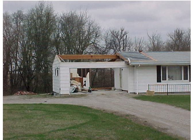
A tornado destroyed the roof and back wall of this garage.
