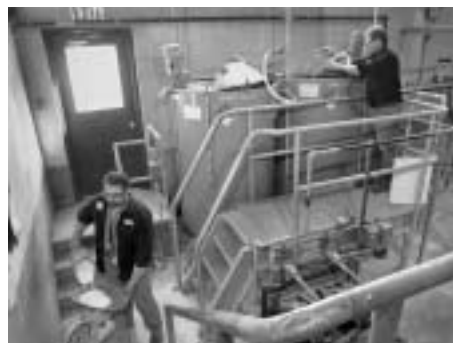
5. POLYMER is also added to the water after aeration to aid in a process called flocculation, whereby very small hydroxide particles stick together to form larger particles, called floc, which are more easily settled and removed (see no. 6). The polymer is mixed with the water in a rapid-mix tank. Steve Barcelo (left) is seen measuring the polymer, while Tom Boucher prepares to mix.
