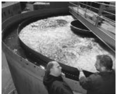
3. AERATION TANK reduces carbon dioxide gas and aids in the oxidation of iron. At the aeration tank, Steve Barcelo (right) describes the action to Frank Masia.
