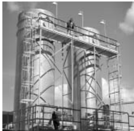
9. AIR-STRIPPING TOWERS remove any volatile organic compounds (VOCs) from the water undergoing the WTF process by spraying the water down over whiffle ball-like fill while air flows upward through the water spray. Inspecting the towers from the top is Steve Barcelo. Frank Masia looks on from below.
