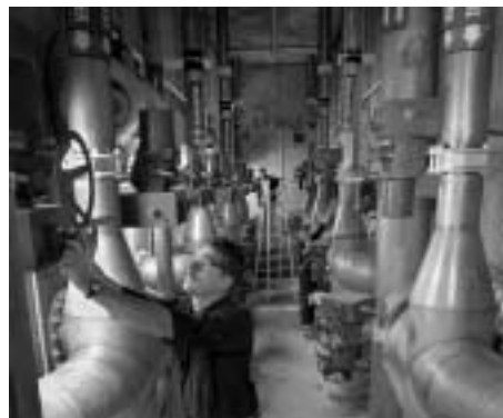
7. FILTRATION is performed, using what is called a rapid sand filter made up of eight filter cells containing sand and anthracite. Inspecting the valves in the filtration valve gallery are: (front to back) Jack Kulesa, Richard Lutz, and Steve Barcelo.
