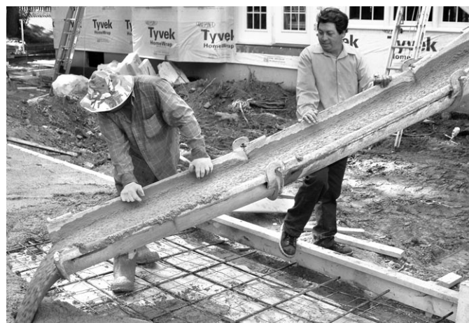
Cement masons first set the forms for holding the concrete and properly align them.
