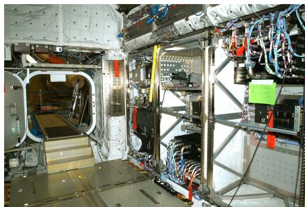
Columbus subsystem racks during testing.
