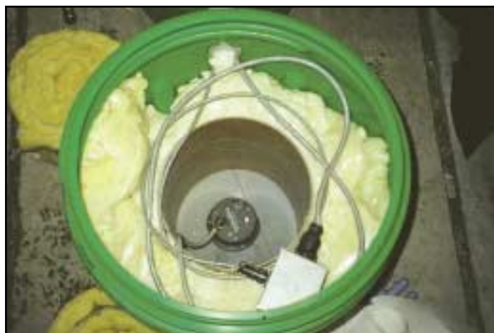
Figure 9. Strong-motion sensor installed.
