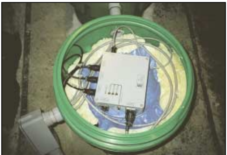
Figure 13. Seismometer feedback electronics connected to seismometers.
