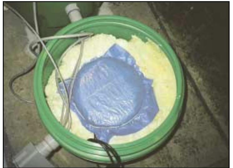
Figure 12. Tarp used to prevent condensation from dripping on insulation.
