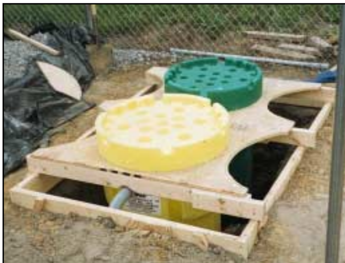
Figure 3a. Barrels in Positioning Jig Station NHSC.
