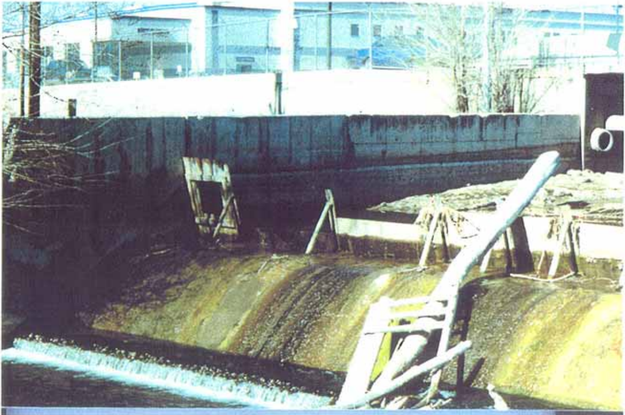
Photo 8-7. Upstream view of Lower City Dam. At the left side of the photo, note the 3-foot-wide metal slot designed to pass 25 cfs.
