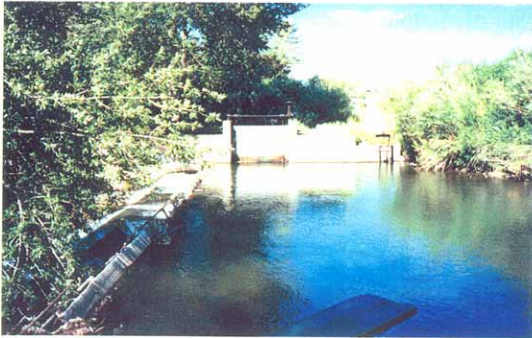
Photo 5-5. Upper Union Diversion: headworks to West Union Canal/West Smith Ditch (large headgate). Small headgate on right is no longer in use.
