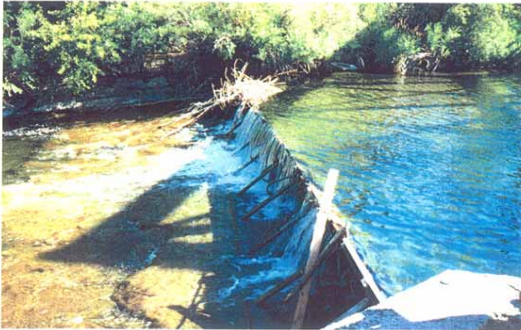
Photo 2-3. Timpanogos Diversion: kick-leg structure.
