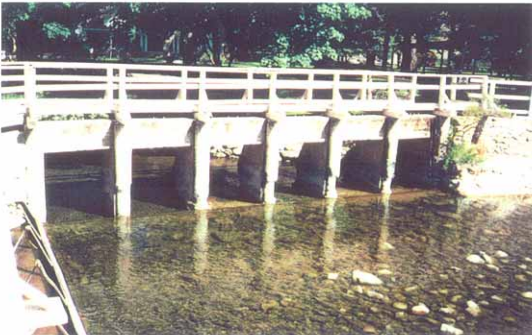
Photo 3-4. Provo Bench - diversion on river: canal head works.
