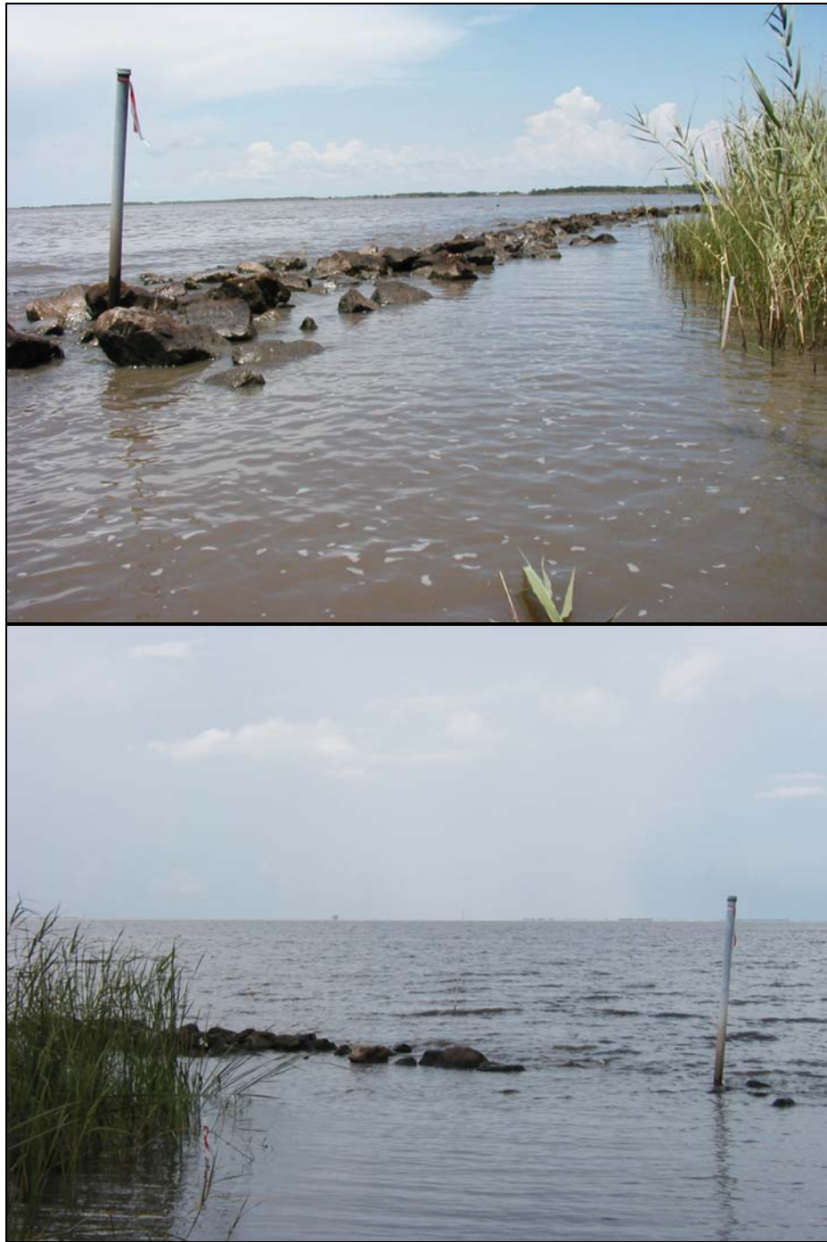
Figure 6. Photograph of rock breakwater and vegetation growth at settlement plate 1005 (upper) and water overtopping rock breakwater at settlement plate 1006 (lower).
