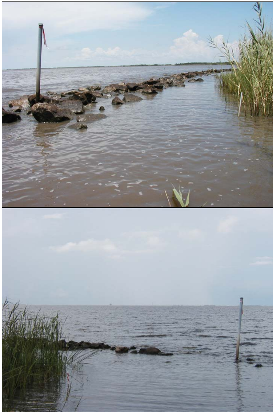
Figure 7. Photograph of rock breakwater and vegetation growth at settlement plate 1005 (upper) and water overtopping rock breakwater at settlement plate 1006, July 2002 (lower).
