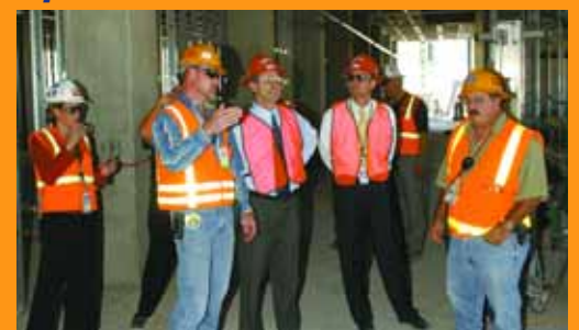
Labs President and Director Tom Hunter does an ES&H walkthrough of the MESA construction project. More Bill Doty photos on page 7.
