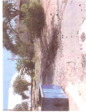
Drainage Problem, Apartments on the North-West corner of Ash and Buena Vista
