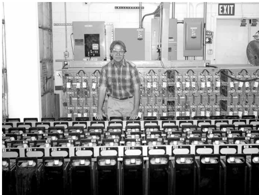
JERRY GINN displays some of Sandia's battery storage capability. Energy storage is an integral part of the Energy Surety Microgrid. (Photo by Bill Doty)
