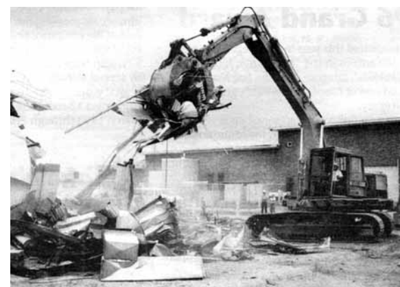
BLDG. 844, one of Sandia's original buildings, meets the wrecking machine in this 1996 photo. The building was erected in either 1946 or 1947.
