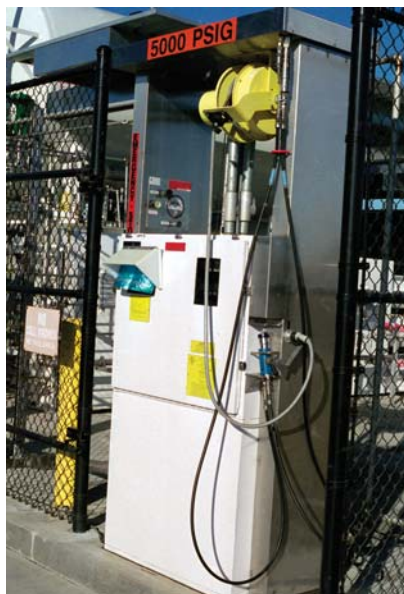
Figure 5-7. A systems approach is needed for integrated hydrogen production, delivery, and storage, as well as for refueling hydrogen vehicles.
