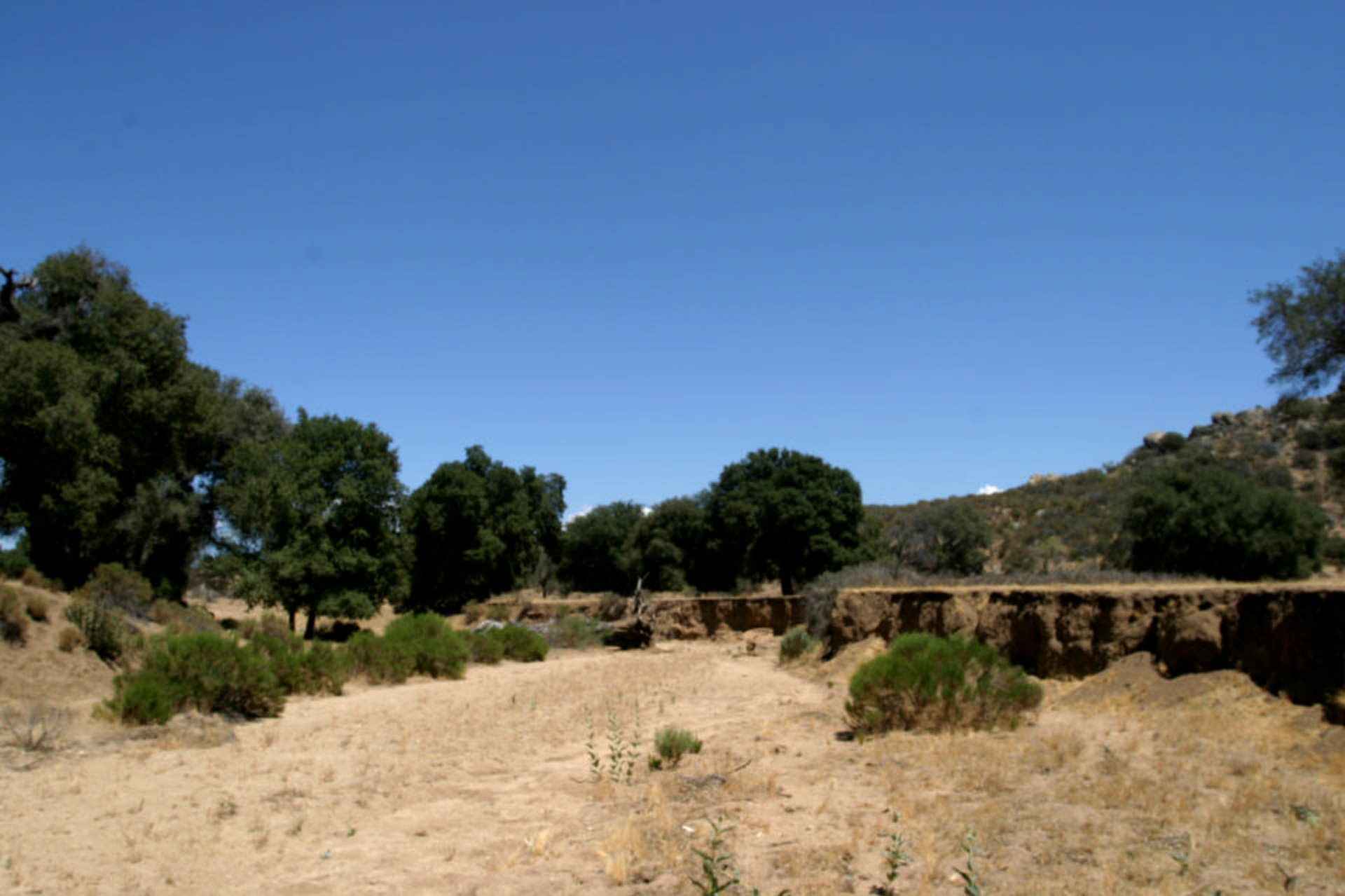
Severe Erosion Near Nejí in the Mexican Part of the Upper TRW
