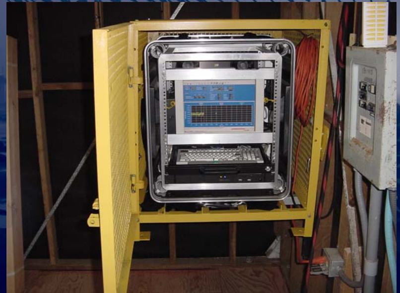
Data Acquisition System
