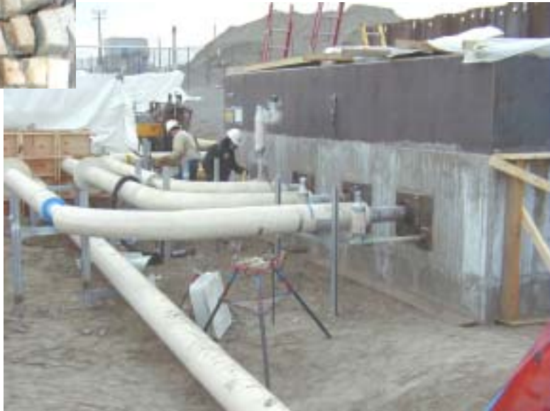
Waste transfer lines are being upgraded in preparation in delivering waste to the treatment facilities.
