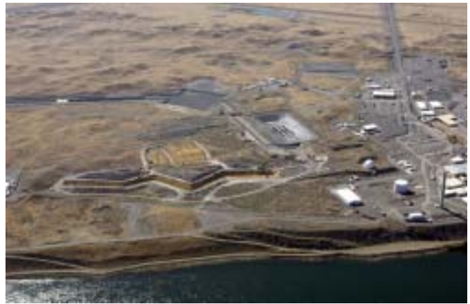
Workers are cleaning up trenches and associated waste sites around the trenches at the 100-N Area.
