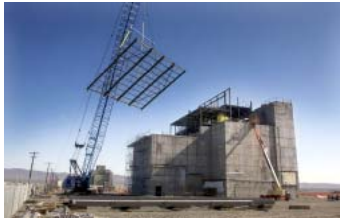
Workers construct a new roof structure to safely enclose the 100-D/R Reactor core; this is the final step in Interim Safe Storage of the core.
