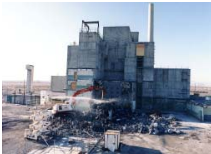
As part of the Interim Safe Storage Project, the control rod room for the 100-DR Reactor is demolished.
