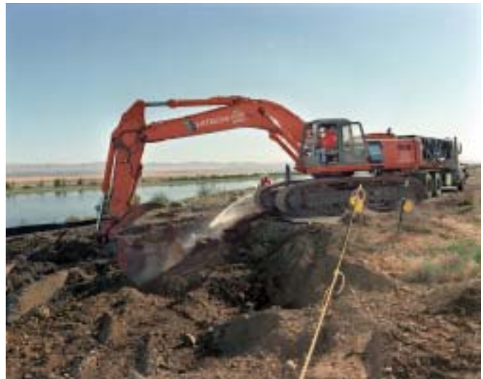
Removing contaminated soil near the retired reactor areas along the Columbia River.
