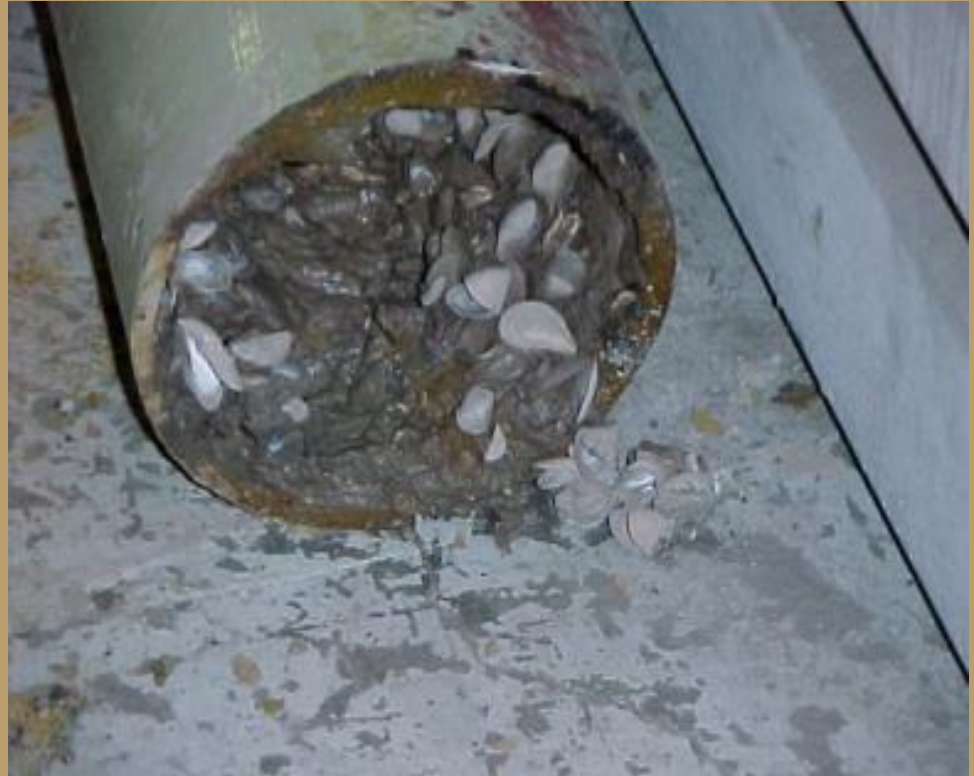
Water Cooled Transformer Piping
