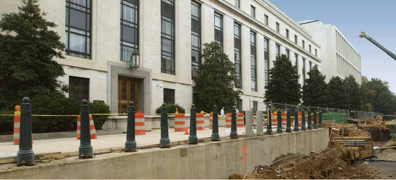
2008 infrastructure improvements included the continued installation of retractable bollards to help provide perimeter security throughout the Capitol complex.
