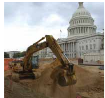
The construction of the historic Capitol Visitor Center proceeded in several phases. Site preparation and tree preservation work started in October 2001.
