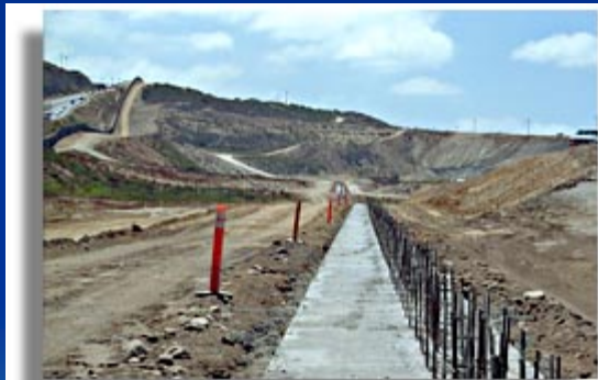
Foundations of a new wall, part of the triple fence being constructed on the border. Click for large version. Photo by Nic Paget-Clarke.
