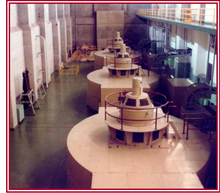
Turbines and Generators
