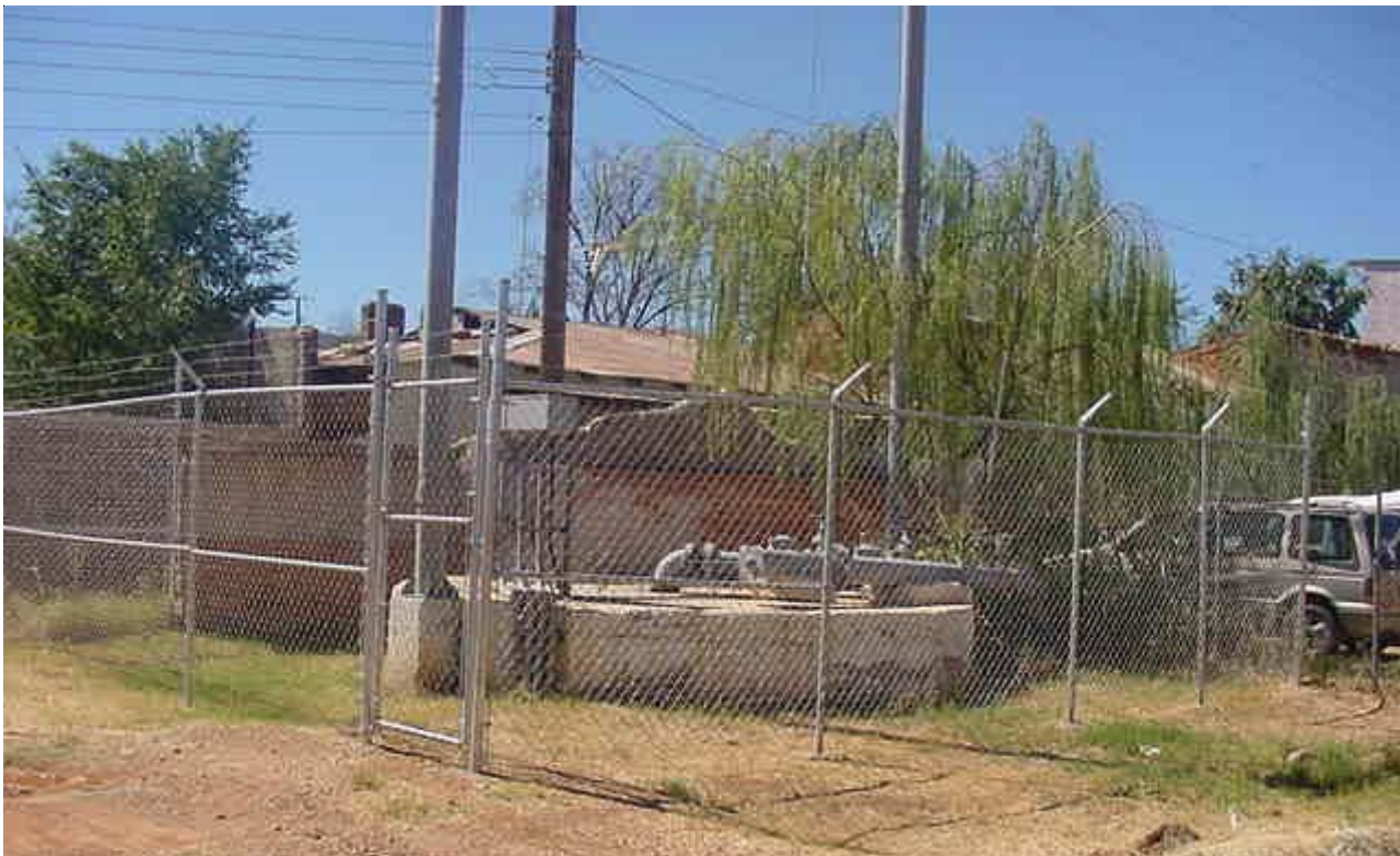
Wastewater infrastructure in Naco, Sonora
