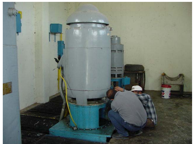
Morillo Drain pump
