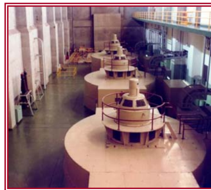
Turbines and Generators
