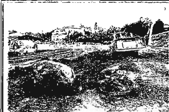
Photo 169 Boulders uncovered during grading operations.
