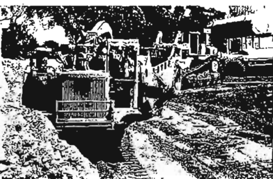
Photo 101 Grading operations near the ash pit excavation. The ash pit is located to the right of the photograph.
