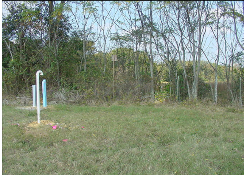
On-site methane ventilation well located within 100 feet of residential property to the east.
