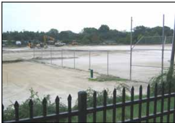
6. After remediation was complete, site restoration activities were conducted for the baseball field in MP. A groundwater monitoring well can be seen in the center of the photograph.
