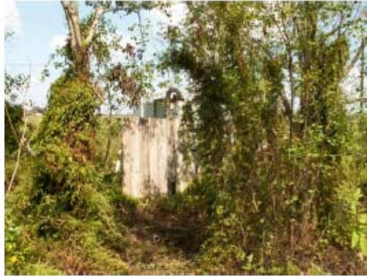
File Name: PAO_photo2.JPG Date/Time Taken: 01 Oct 2005 1258 Description: Sewage treatment structure, showing no storm damage, view to north. N30°01'00.2"; W92°07'19.9"
