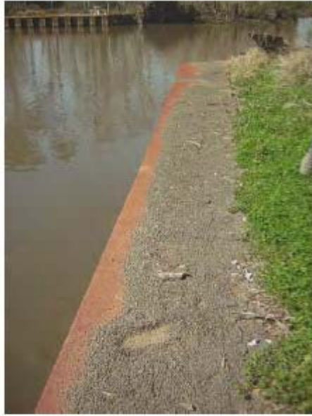
Photo 29: Dried sediment on top of sheet pile wall along bayou left behind by floodwaters associated with Hurricanes Katrina/Rita. Taken 2/16/2006
