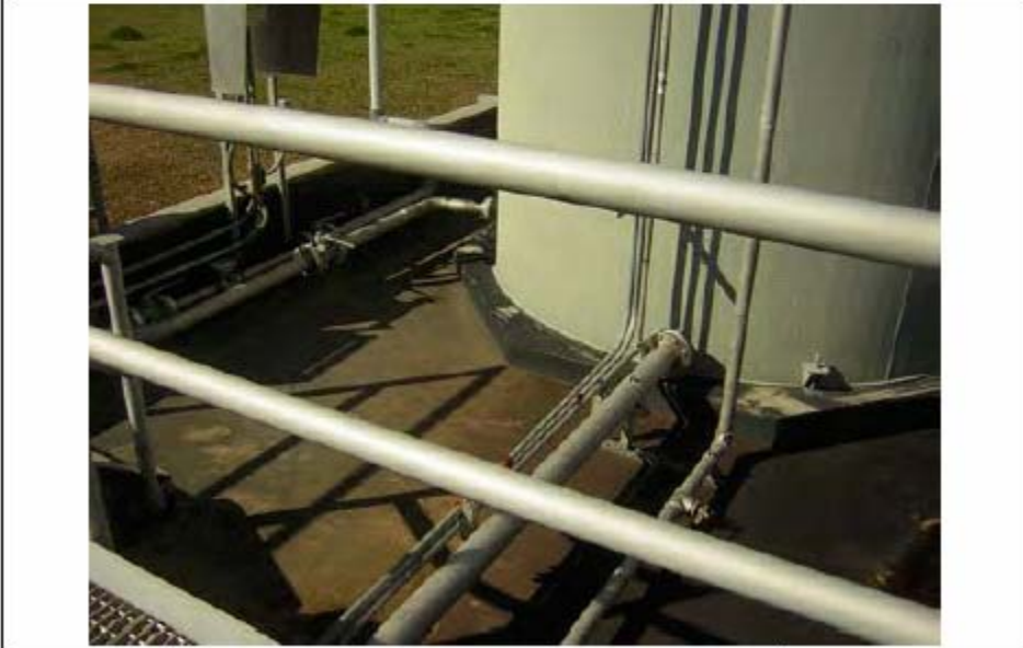
Photo 8: Ground water treatment system piping. Taken 2/16/2006
