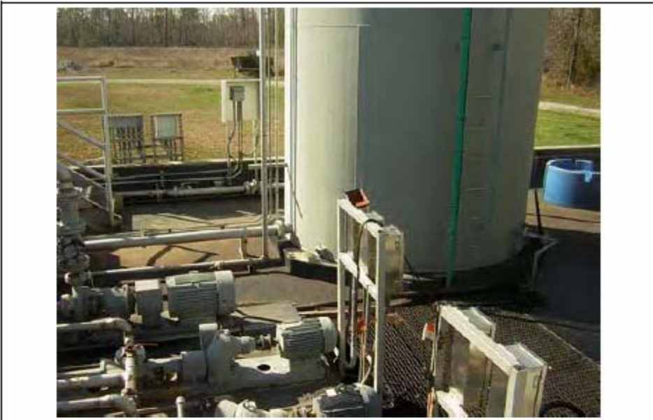
Photo 7: Bottom left, pumps within ground water treatment system, submerged and damaged during Hurricane Katrina. Taken 2/16/2006.
