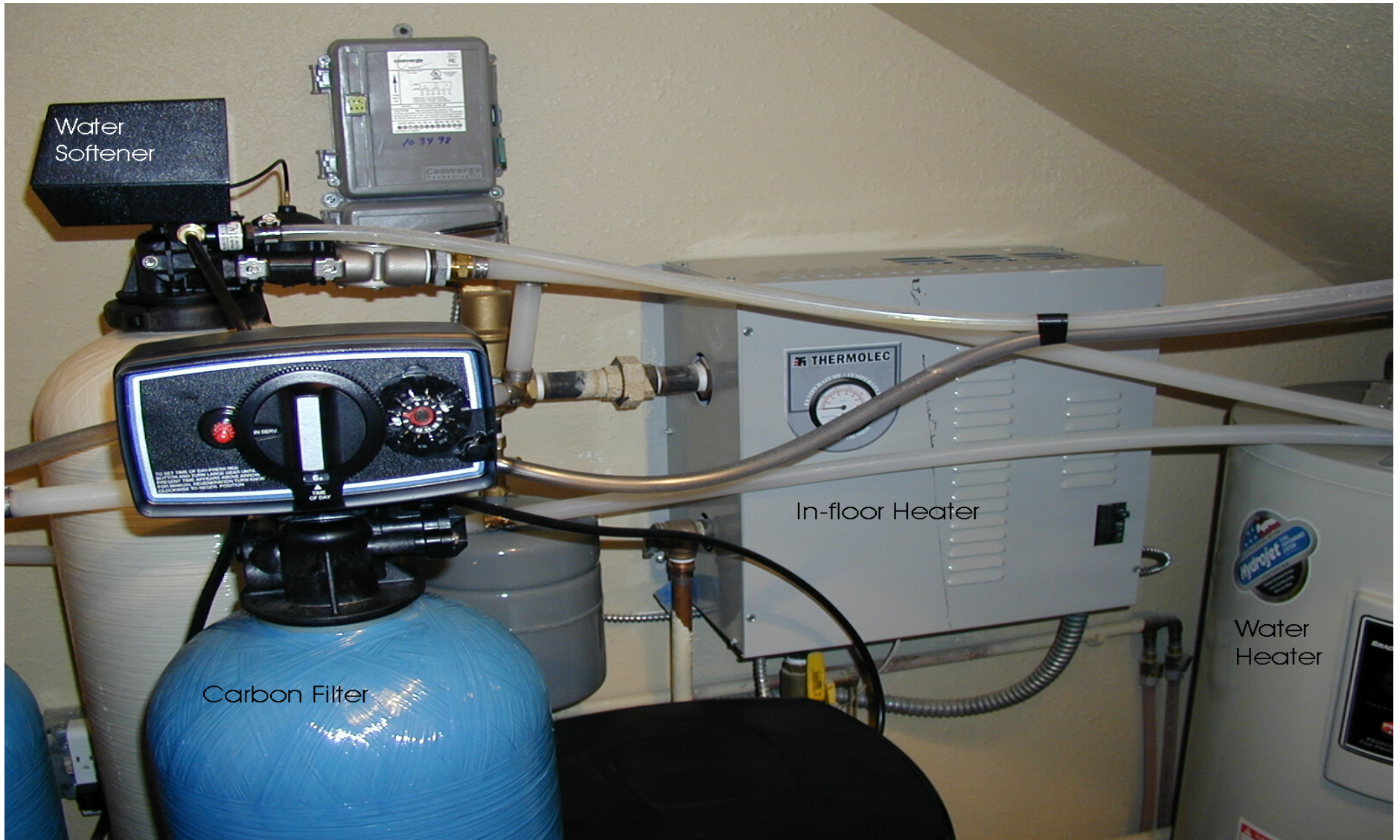
Wintertree Plumbing System.
