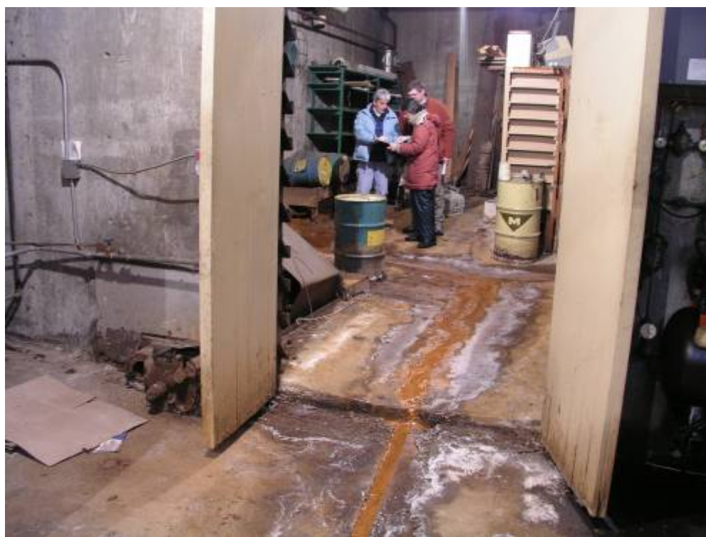
Figure 1: Former Coal Storage Room, Primary School Campus, St. Katharine Drexel School, Beaver Dam, Wisconsin.
