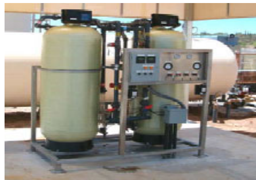
APU-30 System – New River, AZ Arsenic Treatment Project
