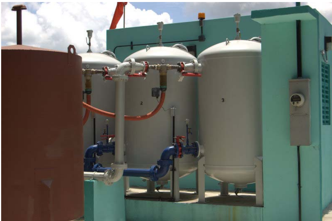
Figure 3 Maunabo Municipal Well #1 Filter Bank
