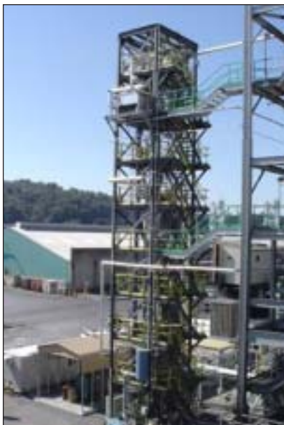
HTDS: High Temperature Desulfurization System installed at the Eastman Chemical Company.
