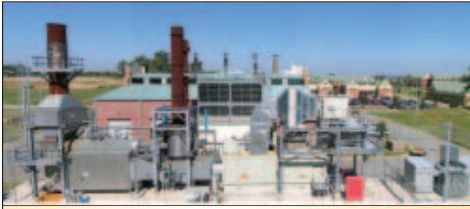
Integrated Energy System: An Integrated Energy system installed at the Fort Bragg 82nd Airborne Central Heating Plant.
