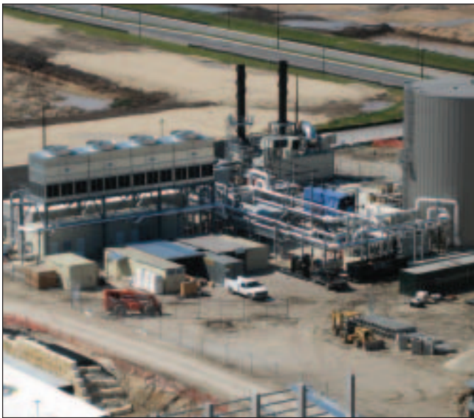
Combined Heat and Power: The new system provides the Dell's Children Hospital 100 percent of the thermal requirements to operate the hospital's power supply; and cleaner, more reliable power that has a power backup to the electric grid.
