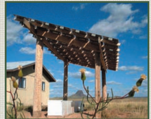
Solar electric array on Navajo home
