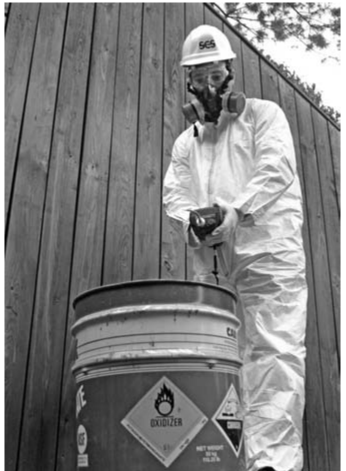
Most hazardous materials removal workers are required to wear respirators to protect them from airborne particles.
