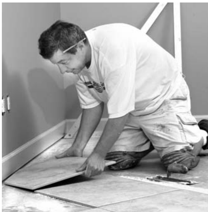
Prior to installing tile, tilesetters use measuring devices and levels to ensure that the tile is placed in a consistent manner.
