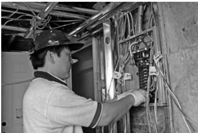
Electricians may rewire a home and replace an old fuse box with a new circuit breaker box to accommodate additional appliances.
