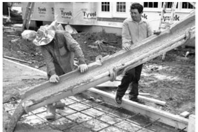
Cement masons first set the forms for holding the concrete and properly align them.
