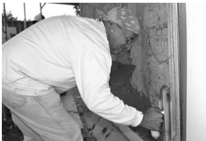
Most plasterers and stucco masons are employed in Florida, Texas, California, and the Southwest, where exterior stucco with decorative finishes is very popular.
