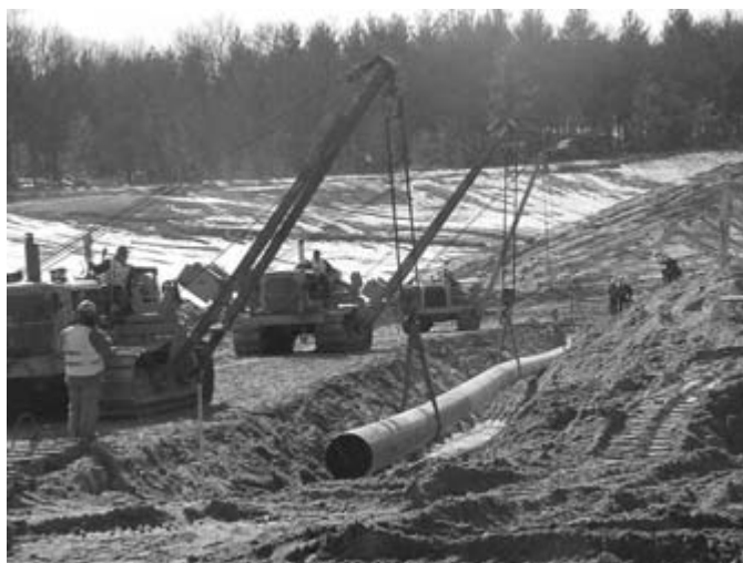
Pipelayers lay clay, concrete, plastic, or cast-iron pipe for drains, sewers, water mains, and oil or gas lines.
