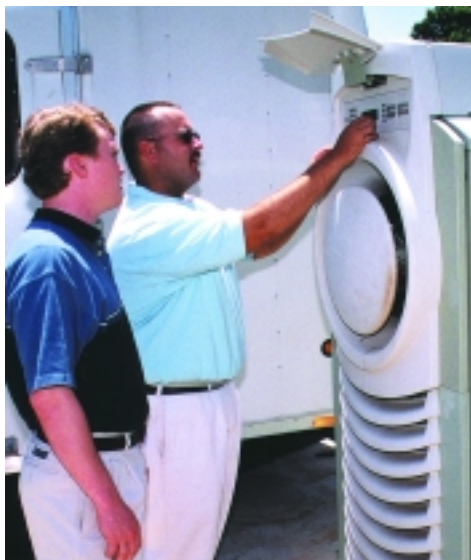
Microturbine power generation is being tested by TVA at some of its facilities.
