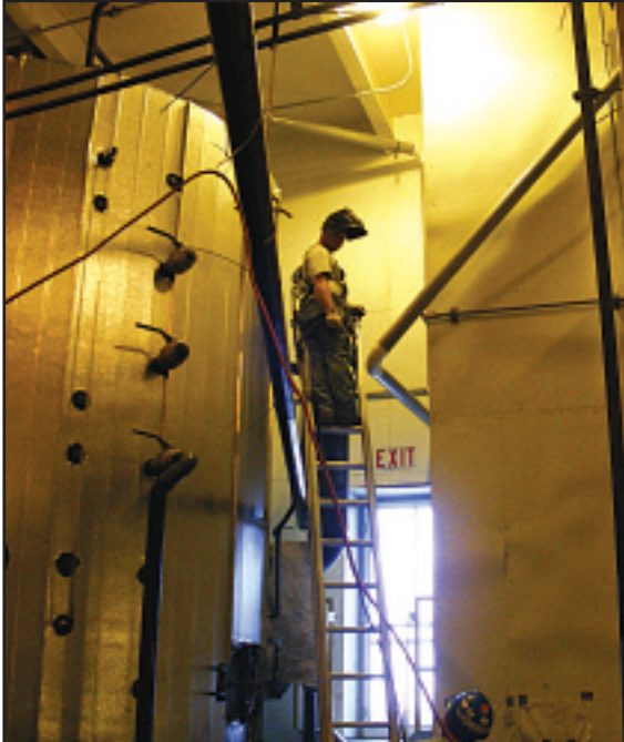
IN A DEMONSTRATION SYSTEM FOR A BIOGASIFICATION PLANT, WORKERS INSTALL A VALVE TO PREVENT UNINTENTIONAL DRAINING. JOHNSON SPACE CENTER IS STUDYING THE FEASIBILITY OF CONSTRUCTING A SIMILAR PLANT TO CONVERT WASTE TO NATURAL GAS.
