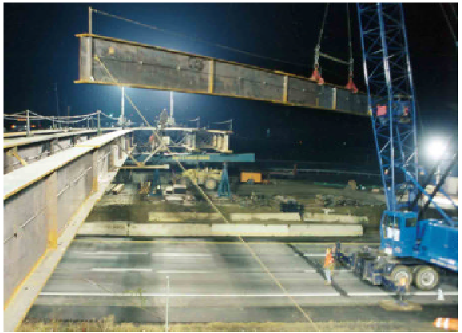
Rifenburg Construction, Inc., adapted VPP for a $28 million highway construction project in New York. Photo by Norm Stahlman
