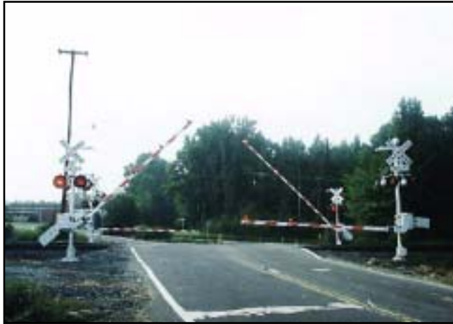
Four Quadrant Gates on the North Carolina Sealed Corridor
