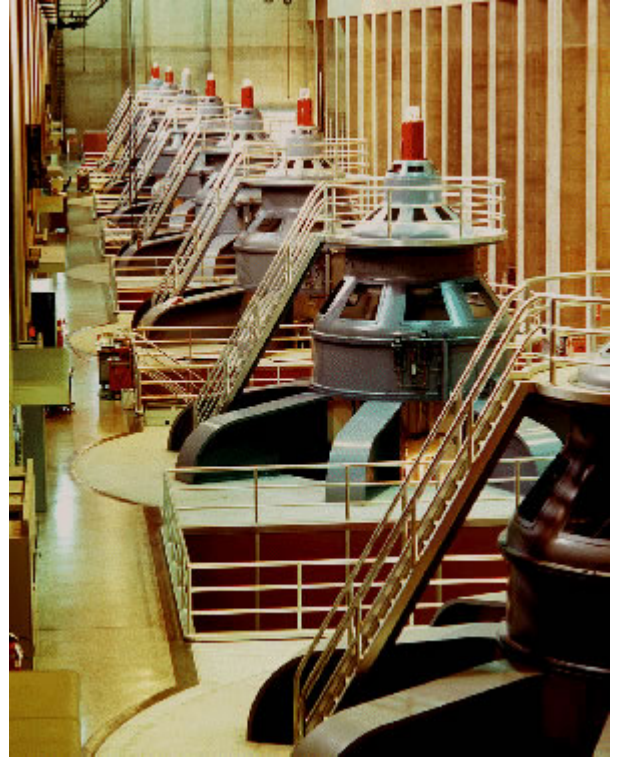
Generators at Hoover Power Plant. Photo Credit: Bureau of Reclamation.
