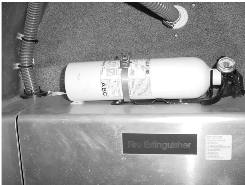
Figure 3-98 B-1 Type Fire Extinguisher
