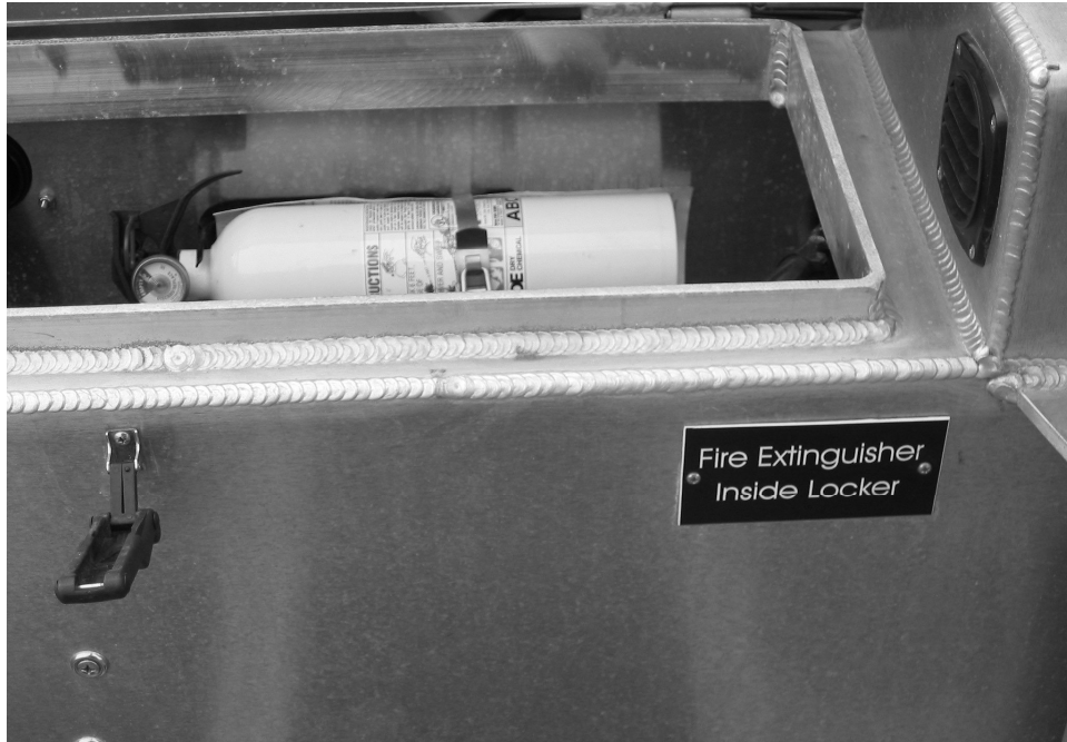
Figure 2-31 Starboard Aft Deck Locker (Defender A Class)
